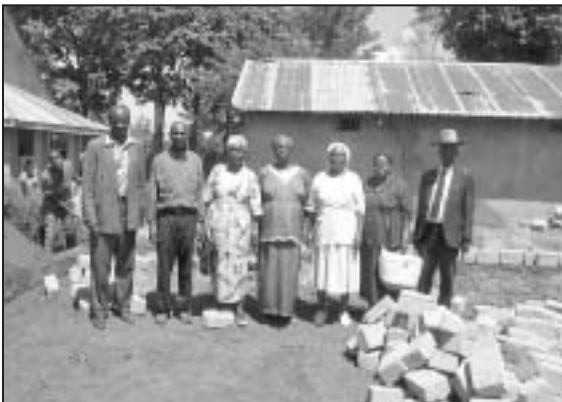
Elders of Kakamega Yearly Meeting amid construction of a dormitory to house and feed AIDS orphans
